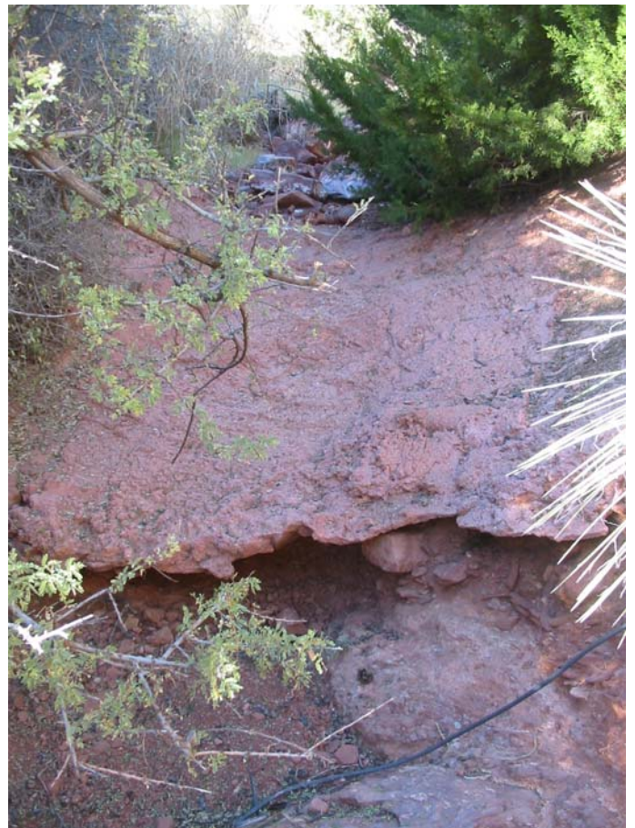
Figure 11b; Photo 2: Failed erosion protection - undercut shotcrete in the vicinity of HW3-S04.
