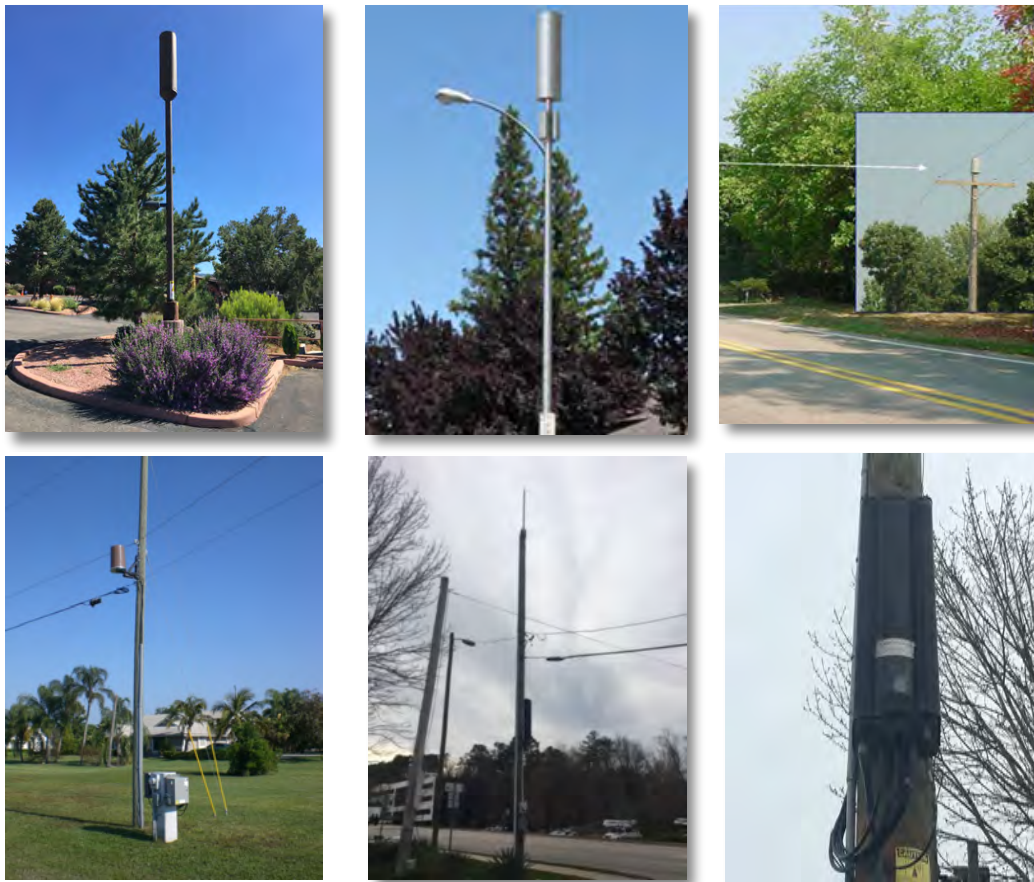
Figure 10: Small Cell Facilities - Single Node
