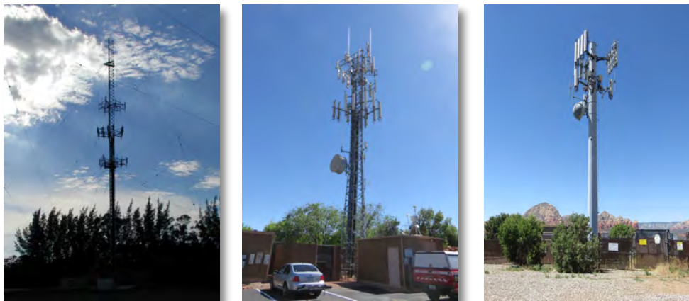
Figure 4: Non-concealed Macro Towers - Guyed - Lattice - Monopole
