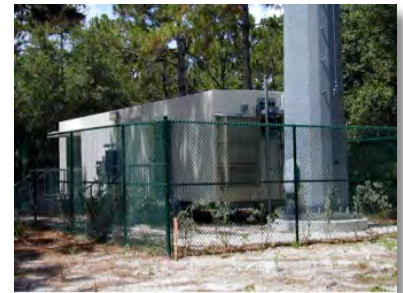
Figure 8: Low Band Facility
