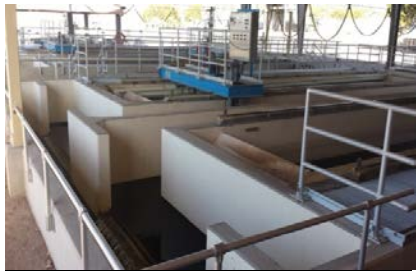
WWRP Tertiary Filters
