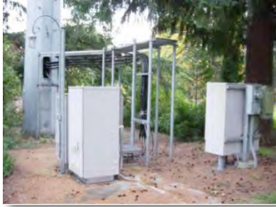
Figure 7: High Band Facility
