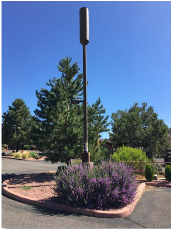
Dual Purpose Concealed Small Cell Facility Red Rocks Church
