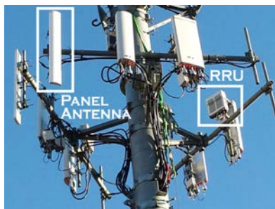
Figure 2: Panel Antennas with RRU's
