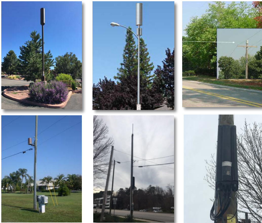
Figure 10: Small Cell Facilities - Single Node
