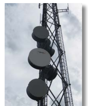
Figure 3: Microwave Dish Antennas
