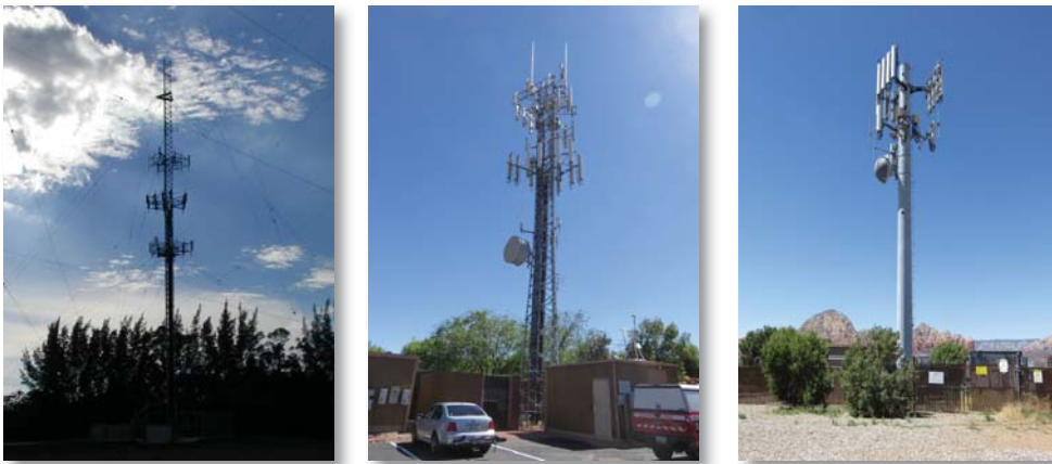
Figure 4: Non-concealed Macro Towers - Guyed - Lattice - Monopole
