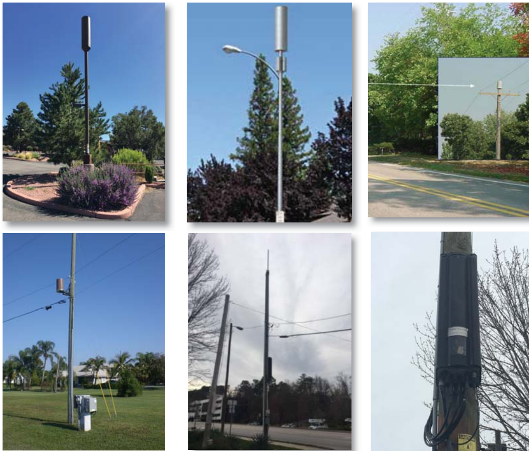
Figure 10: Small Cell Facilities - Single Node
