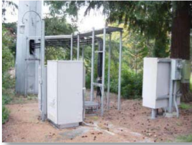
Figure 7: High Band Facility
