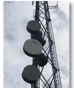
Figure 3: Microwave Dish Antennas
