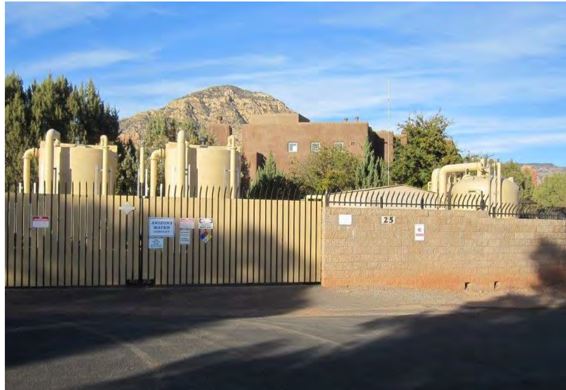
Southwest Center Well No. 8 and arsenic treatment plant a few feet from Adobe Grand Villas and down the street from City Hall.
