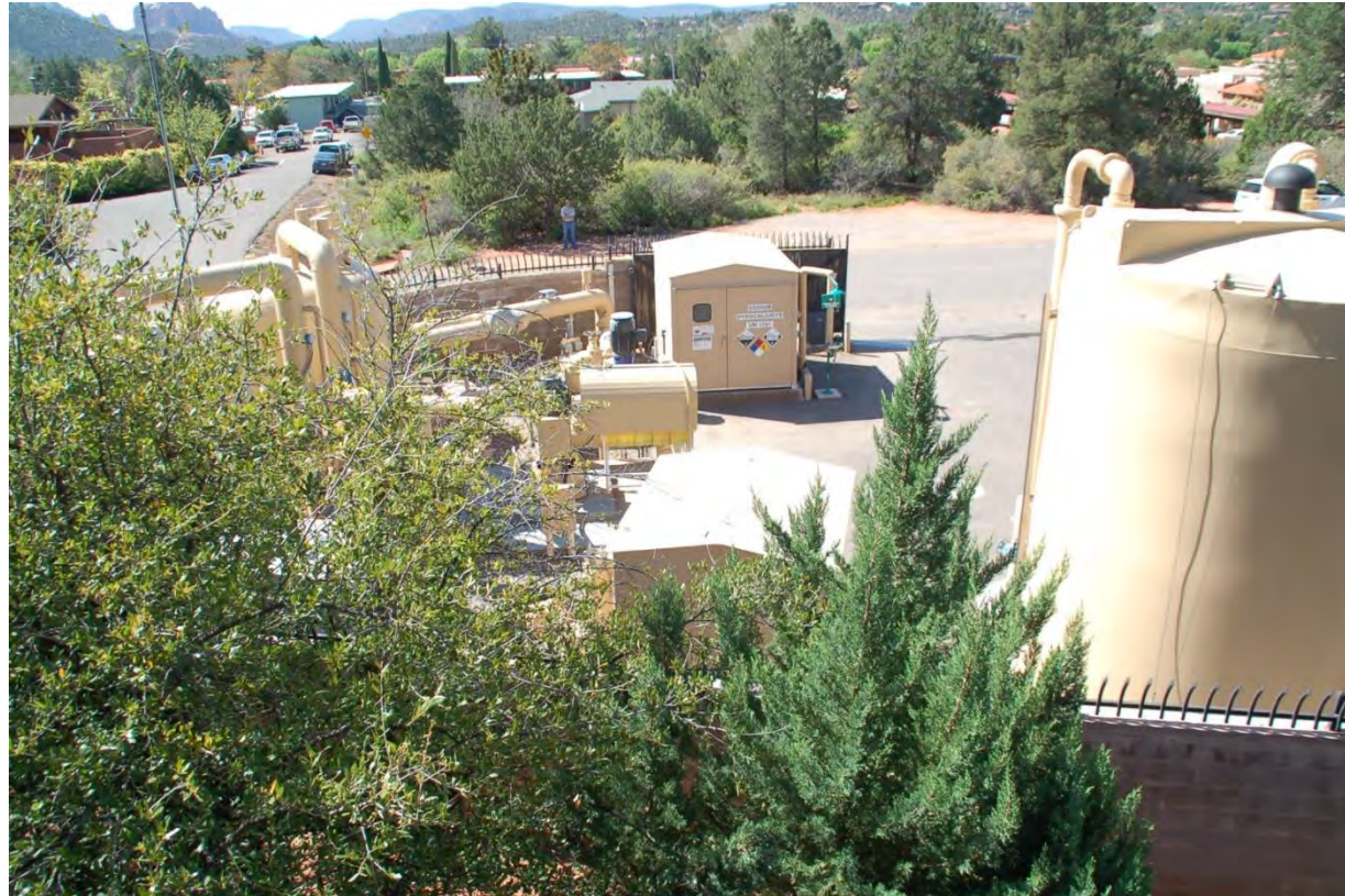
View of well and arsenic treatment system and work yard from the Adobe Grand Villas 2 nd floor.
