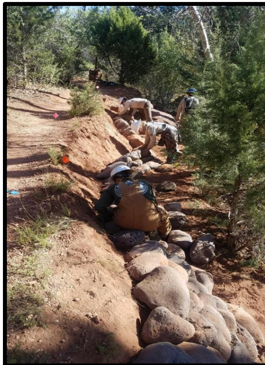
ACE crew installing a six-tiered rock retaining wall on the Allen's Bend trail.
