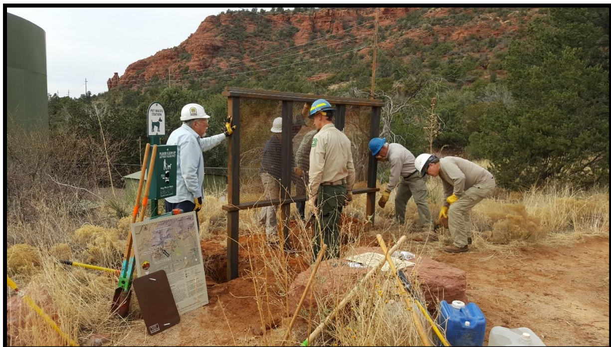
Friends of the Forest completed the install of 12 new kiosks in 2018 including this one at the Andante trailhead.
