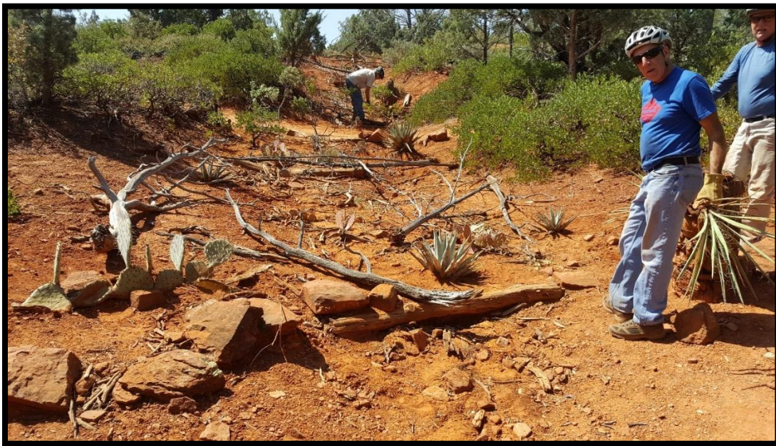
Volunteers at the public work events performing rehab and maintenance on the Jordan trail.
