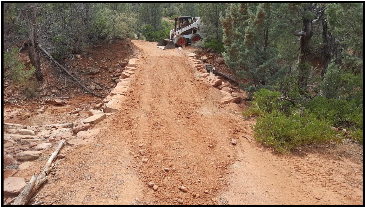
Large culverts needed more material brought in to build up the tread surface.
