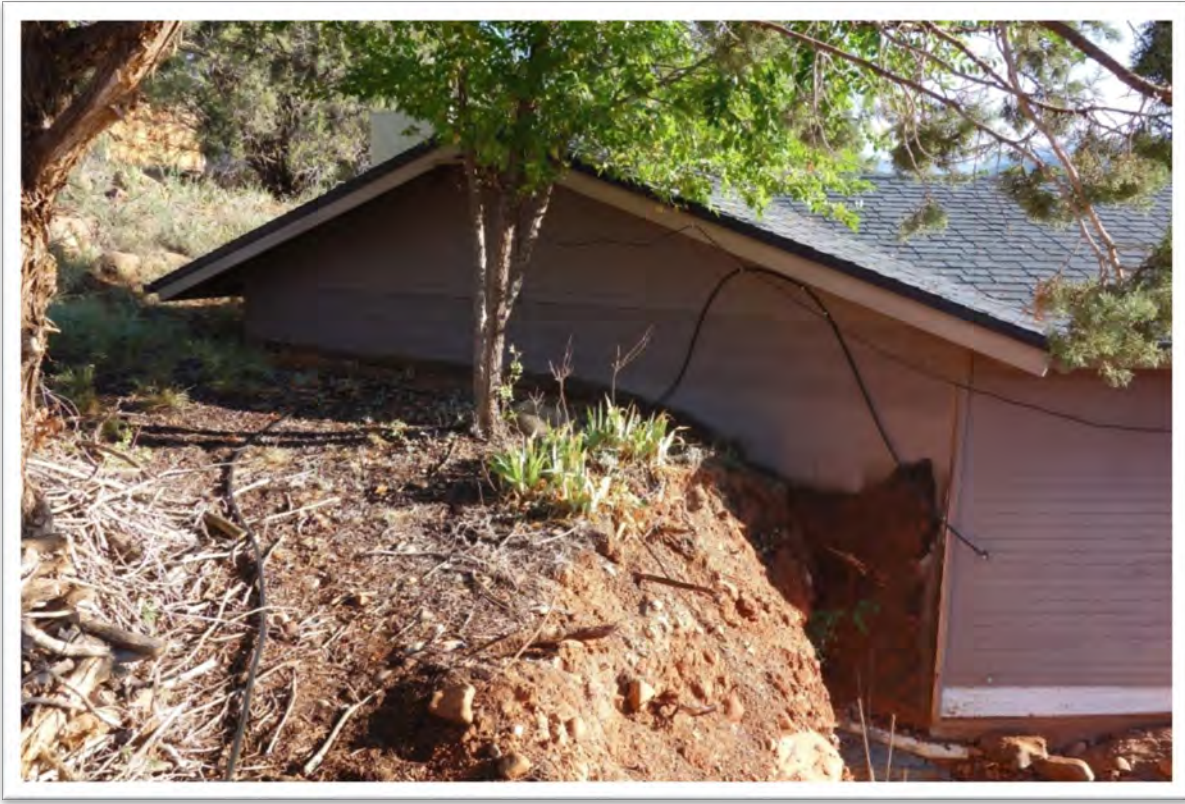
Figure 9: View of the garage from the west, showing the grade difference at the rear property line.
