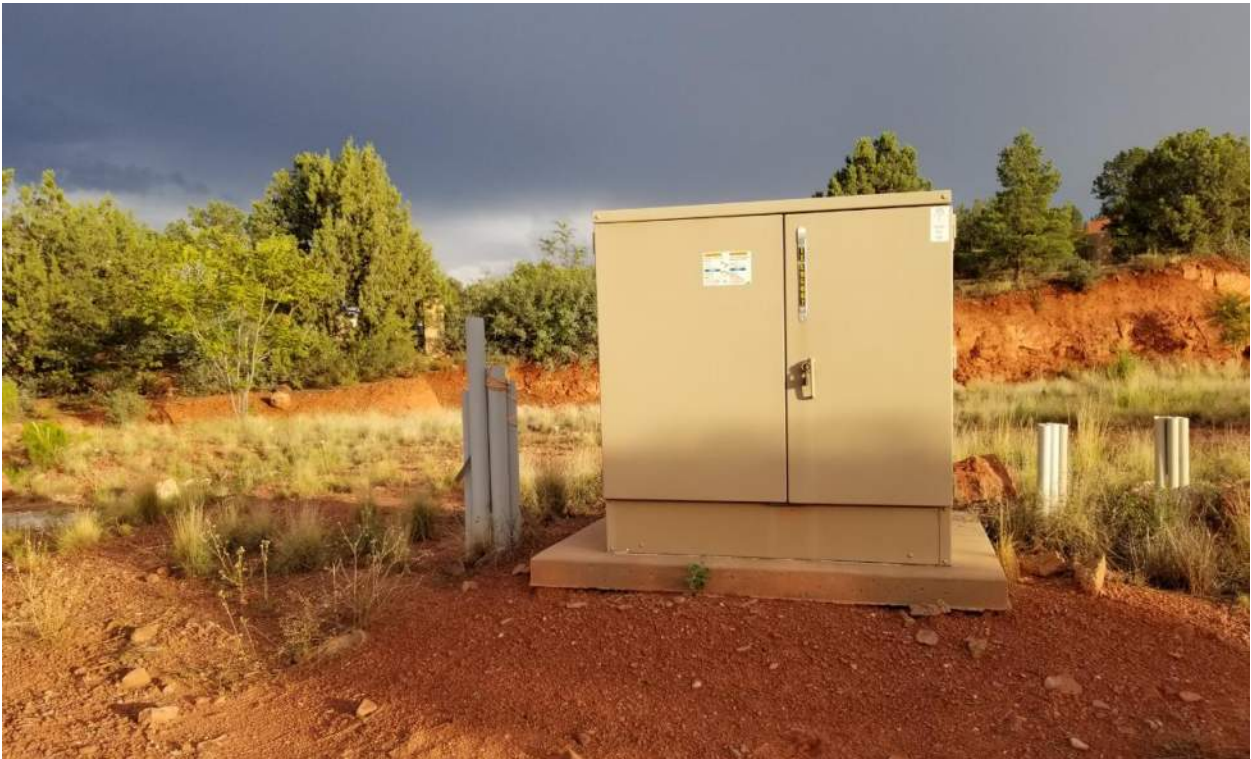
All utilities for the planned original Condominium project are installed and stubbed to the pad locations onsite.
