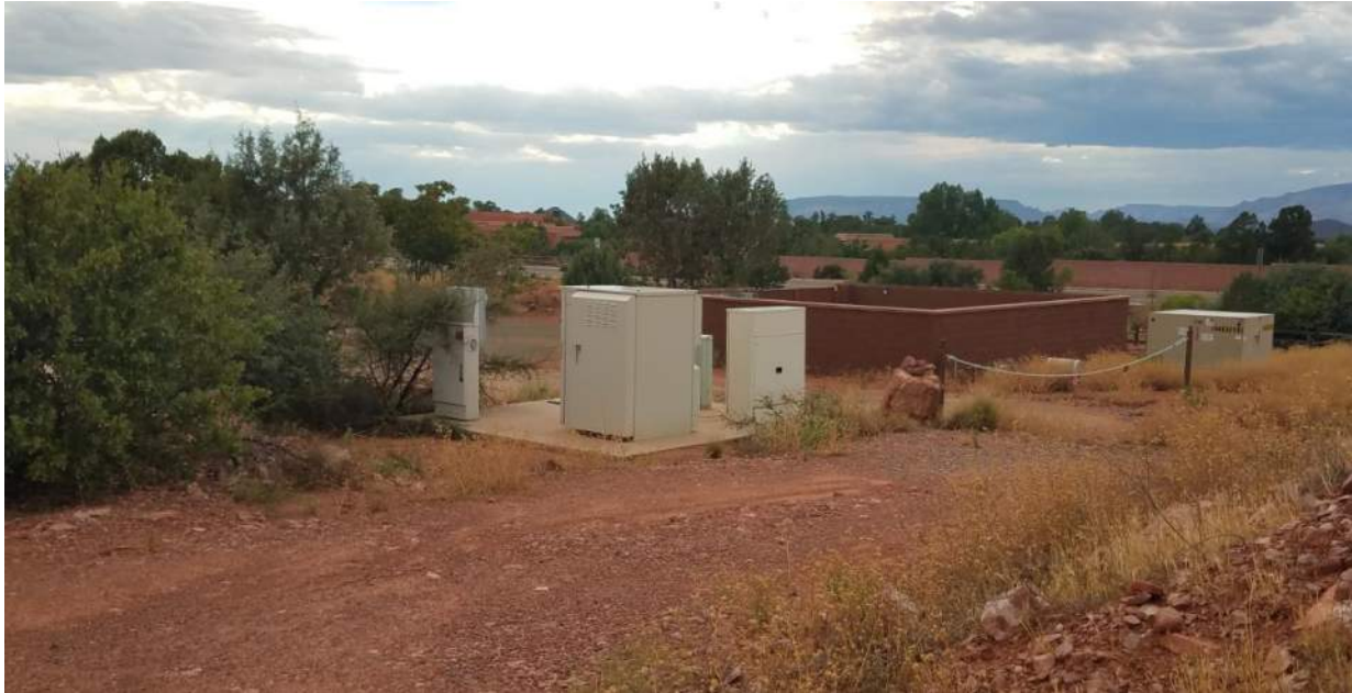
Utilities located at the southwest corner at the shared property line with the Marriott Residence in project within a utility easement.
