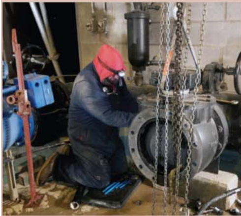
COLLECTIONS OPERATOR WADE WEST WORKS ON A VALVE AT THE CAROLL CANYON LIFT STATION
