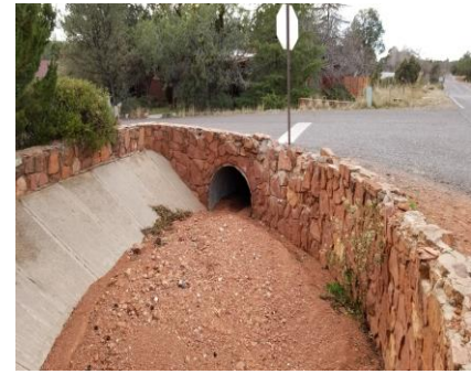
Thunder Mountain Road Undersized Culvert
