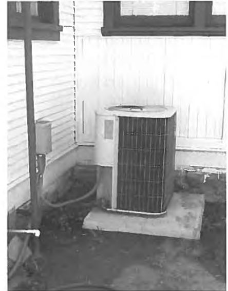
Ranger Residence A/C compressor
