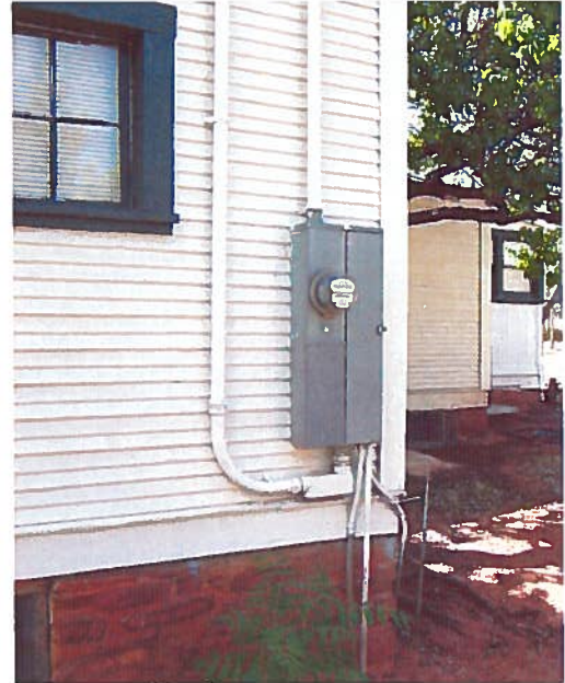
Electrical meter - Ranger Residence
