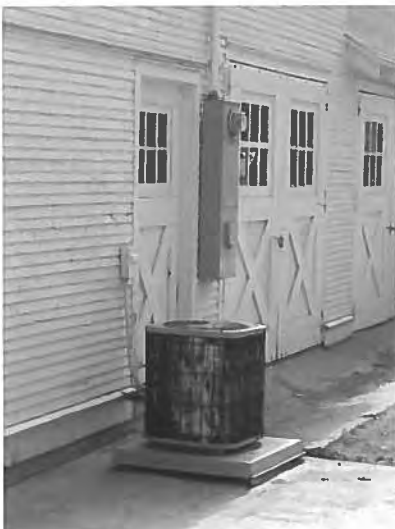
A/C compressor at the Barn
