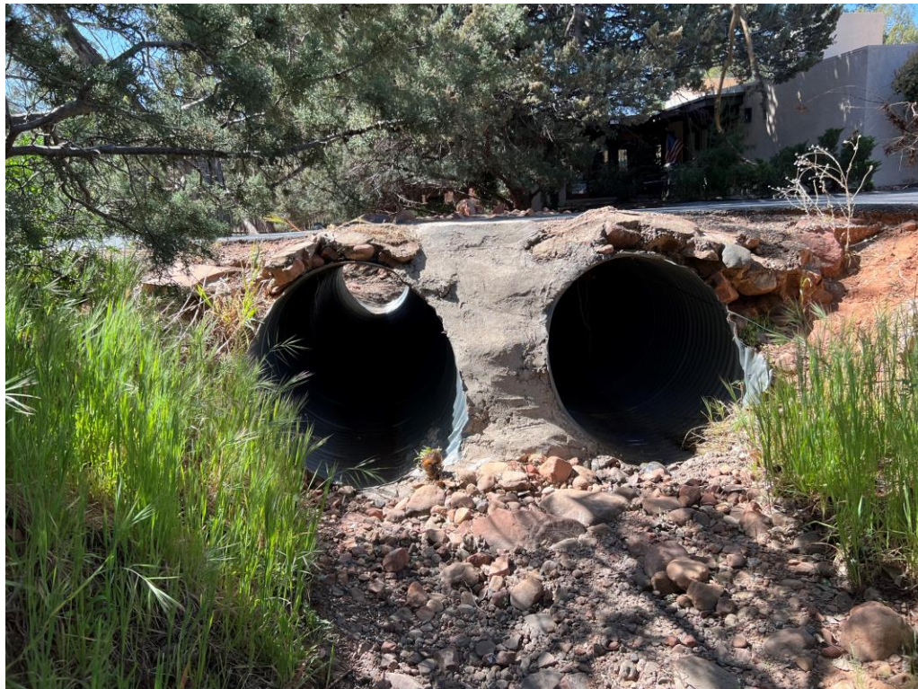
Photograph 4 – Downstream Grade Control at Private Drive
