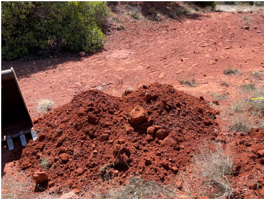
Photo 14 – View of material excavated from Test Pit 7 over the depth range of 0.0 to 1.0 feet, which appears to be primarily excavated native soil over the mudstone bedrock.
