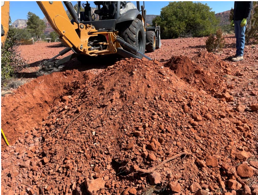
Photo 2 – View of material excavated from Test Pit 1 over the depth range of 0.0 to 4.0 feet.
