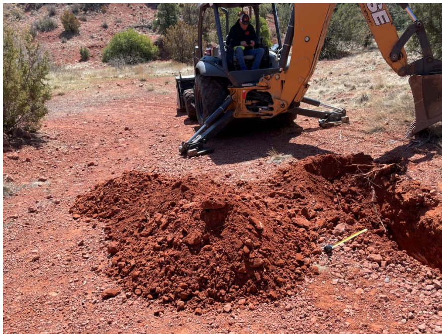
Photo 8 – View of material excavated from Test Pit 4 over the depth range of 0.0 to 2.0 feet, which appears to primarily native soils over the mudstone bedrock.
