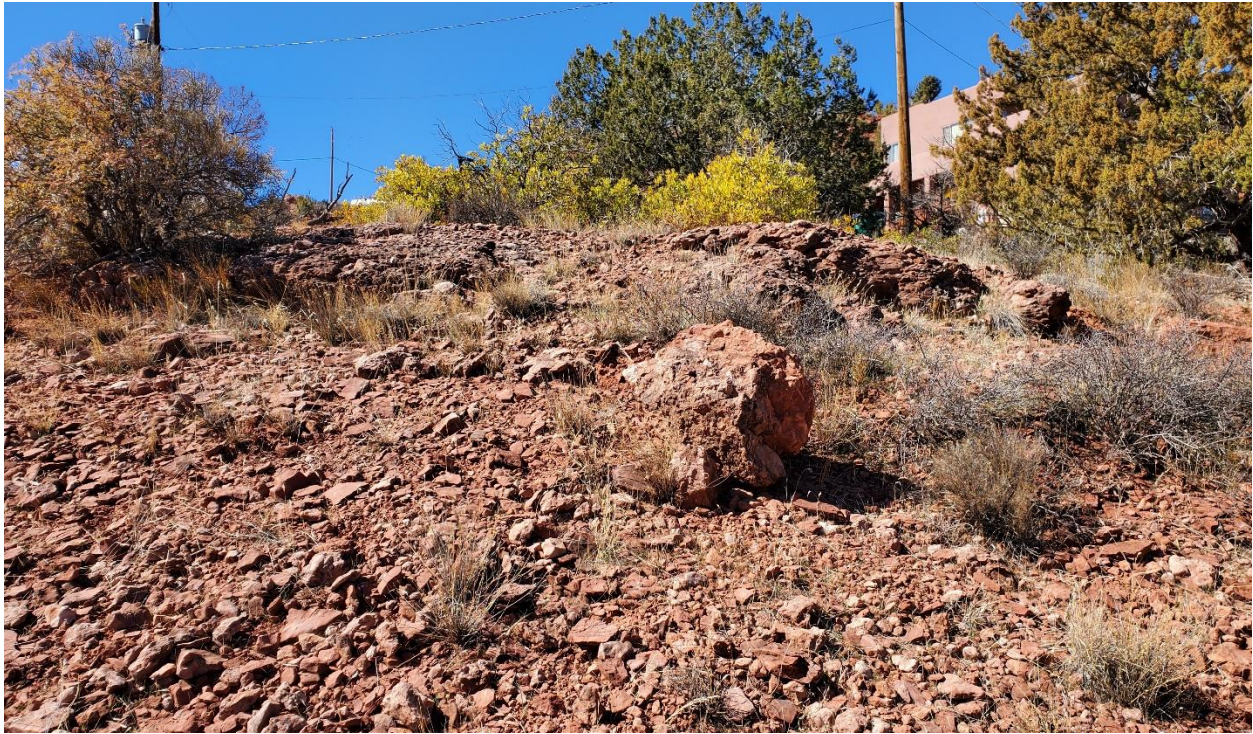
Figure 3: General site conditions showing over-sized aggregate (particles greater than 3.0 inches) and rock outcrops
