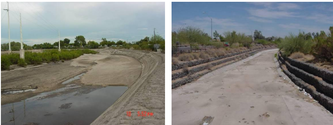
Figure 3. Stream channelization and bank stabilization structures along two rivers in Arizona (photos courtesy of G. Zaines (left) and D. Green (right)).
