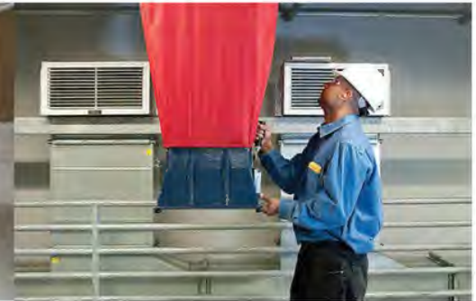
Test and balance (City Hall and WWTP)
