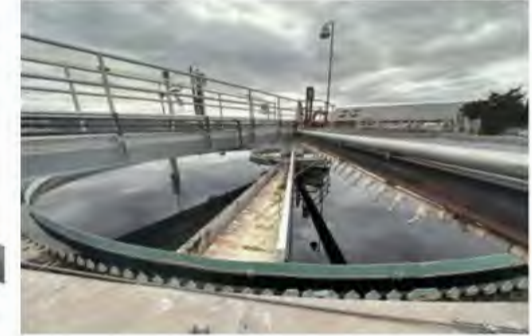
Wastewater Treatment Plant efficient operations
