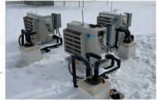
HVAC Roof Top Unit Electrification
