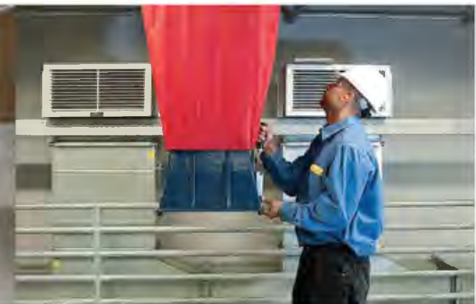
Test and balance (City Hall and WWTP)
