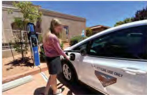
Passenger EV Chargers @ City Hall, Brewer Rd, PW, WWTP
