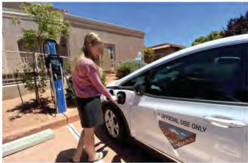
Passenger EV Chargers @ City Hall, Brewer Rd, PW, WWTP
